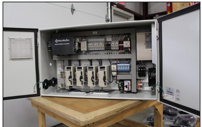
Industrial Router Drive Enclosure
